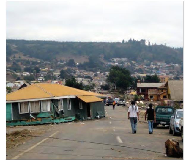
The 2010 Chile Earthquake triggered a tsunami that washed this house in Pelluhue off its foundation and into the street. (Courtesy Caritas Chile)
